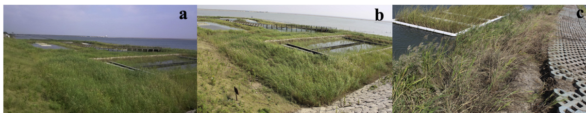
Fig. 6. The appearance of wetland after typhoon landing. a) The overview of the wetland before typhoon Fung-wong; b) The overview of the wetland after typhoon Vongfong; c) Erosion caused by the tide and typhoon-induced storm surge.
